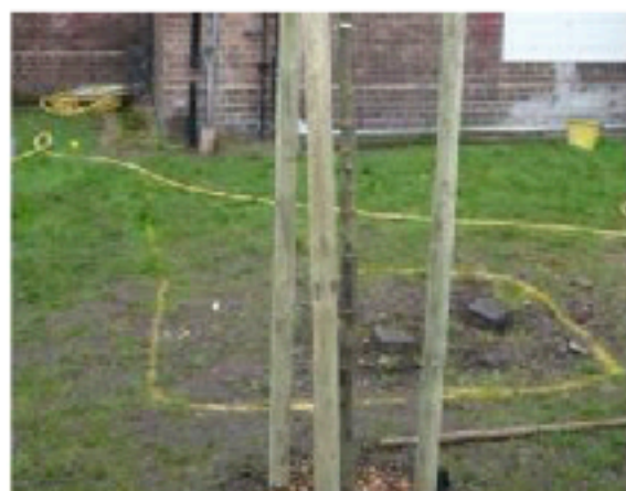
image: recently planted tree and rain garden redesigned around the underground services
